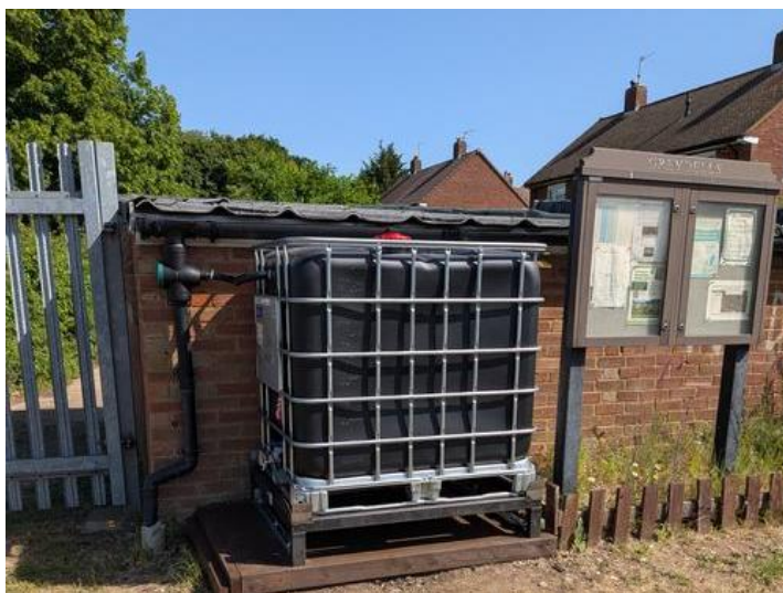
Figure 29. Greydells allotments rainwater harvesting project.
